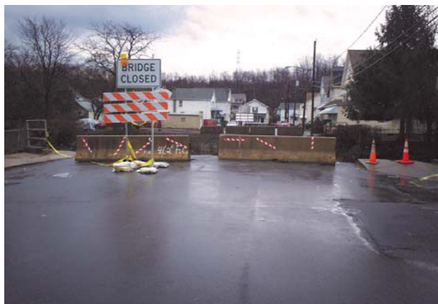
Site of the washed-away Cleveland St. Bridge
